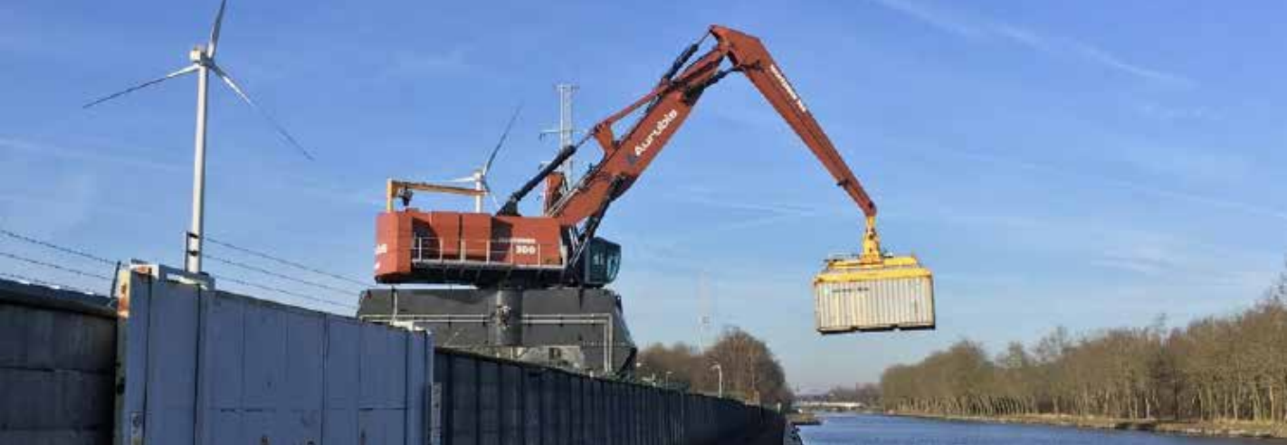
Initial test runs in the ship loading facility (Cu-Port) at the Olen site
