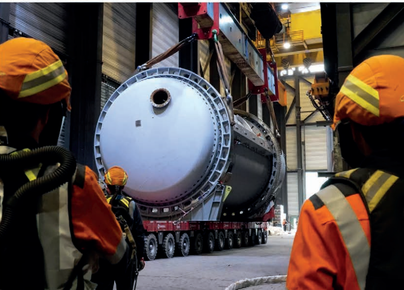
Hydrogen-ready anode furnaces installed at the Hamburg site.
